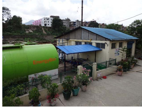
Figure 4.41 New waste-to-energy plant in Teku
