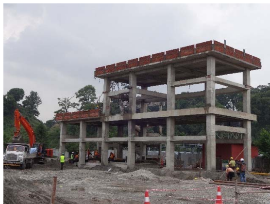
Figure 4.35 Construction of new centrifuge as part of Guheshowri expansion project Source: (R Dewhurst 2017)
