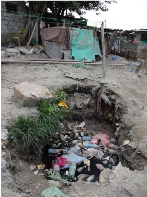
Figure 4.32 Severed toilet pipe discharging blackwater directly into the environment
